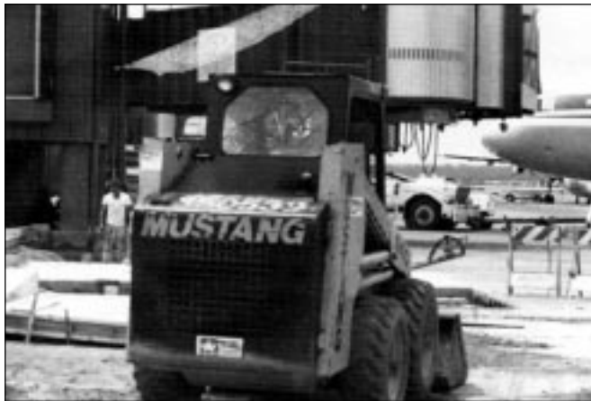
Construction operators must plan movements of mobile equipment to keep within designated work areas and avoid conflict with nearby aircraft operations.
