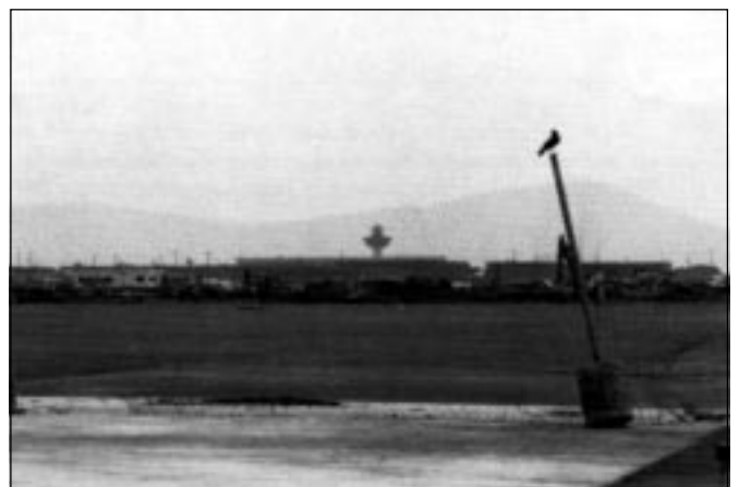
Temporary fencing separates airport and construction activities and can easily be adjusted to conform to changing shapes of work areas.
