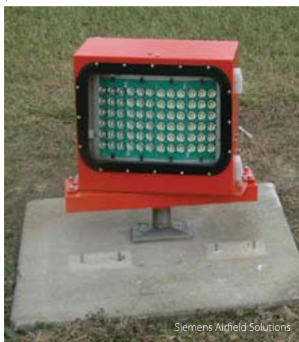
LED runway end identifier lights.
